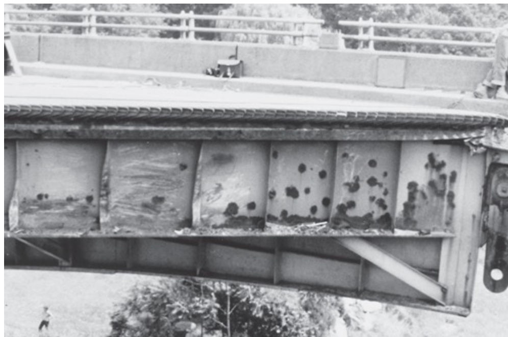
Figure 2.1 Mianus River Bridge collapse (Connor et al. 2005)
